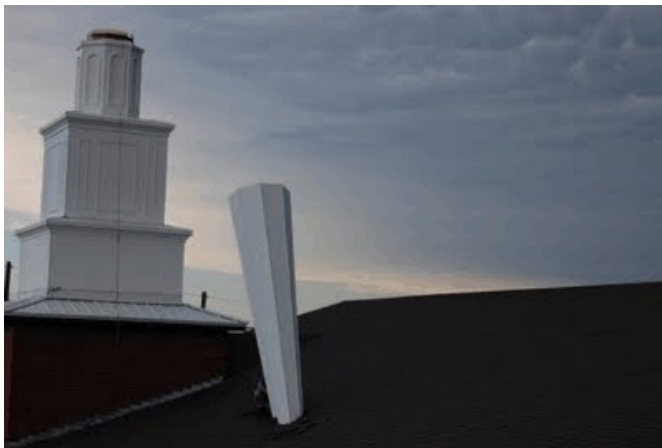
Salina Kansas, First Baptist Church Storm Damage
